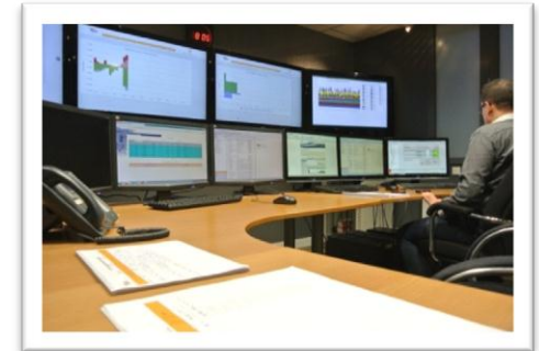
24/7 Network Operation Center in Chambéry
